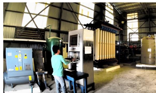
Figure 12. Water Filtration Plant
