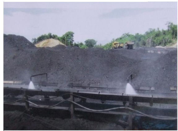
Figure 3. Water sprinkle along conveyor belt
